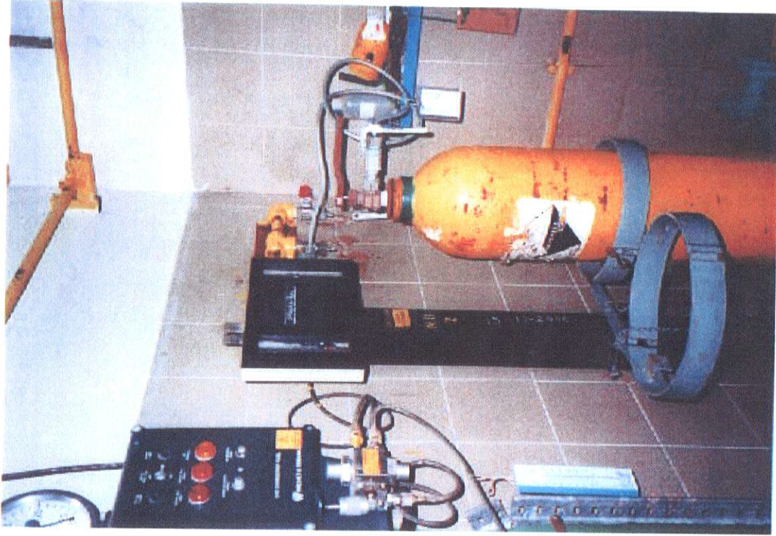
Photograph 4 : Draw-off Point in Chlorination Room 2
