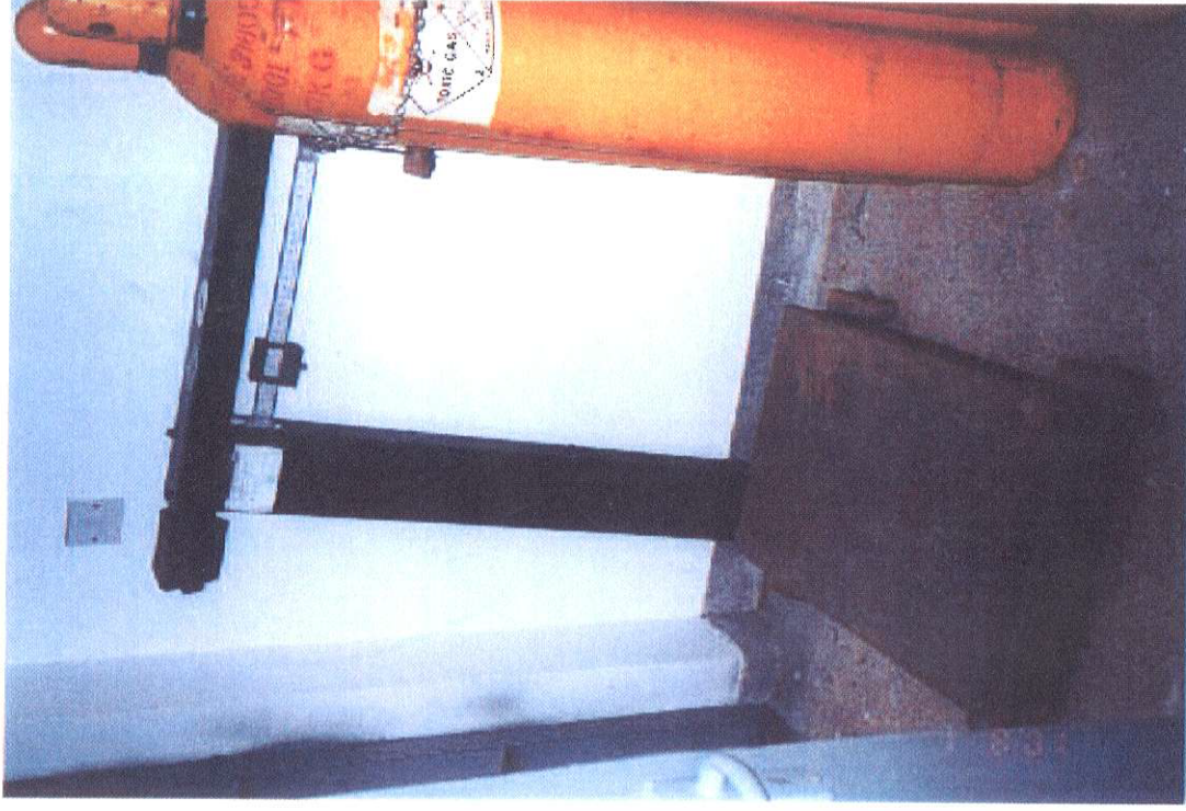
Photograph 2 : Weighscales in Hydrant Chlorine Store
