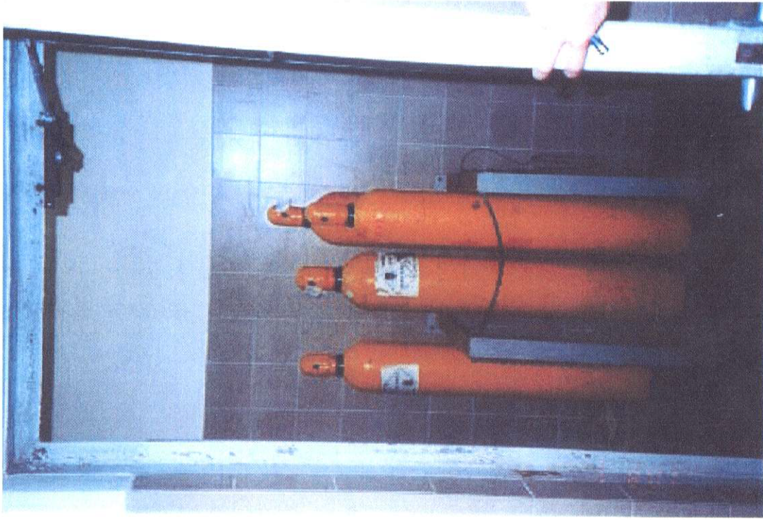
Photograph 1 : Cylinders in Hydrant Chlorine Store
